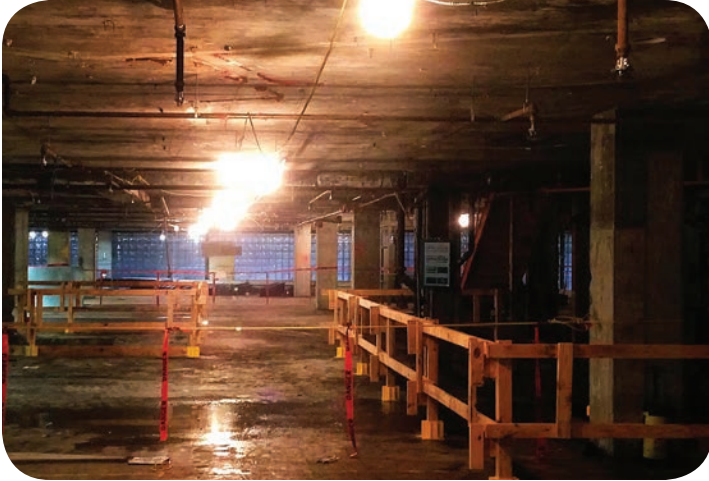
Traditional 100W incandescent system left onsite by demolition contractor
