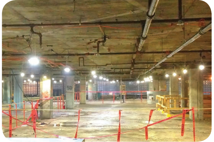
FLEX SLS LED System as installed by construction manager and electrical contractor
